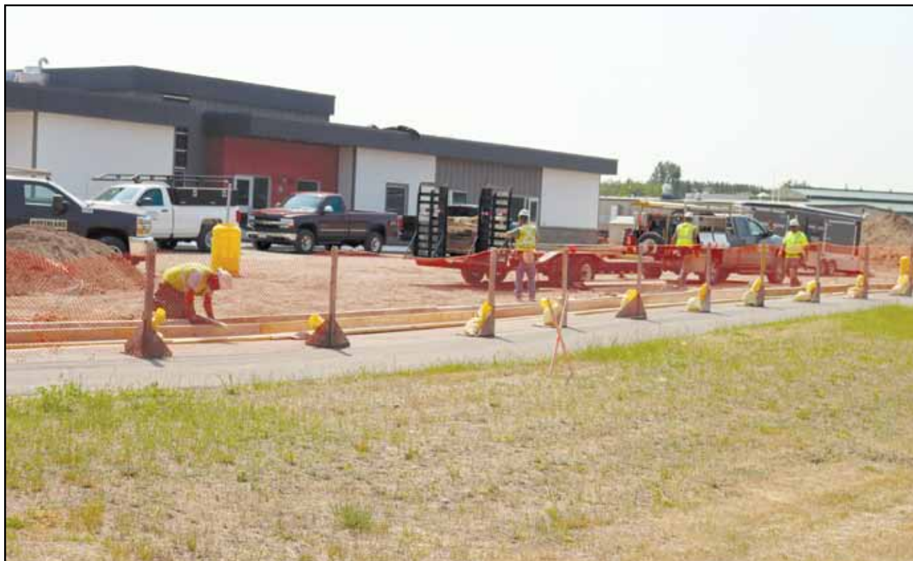
The crew hard at work putting in the parking lot for FDL's new day care facility.
